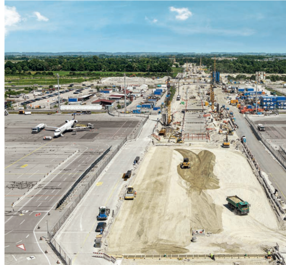
View from the apron tower in the satellite building to the east over the construction works for the suburban rail tunnel to Erding
